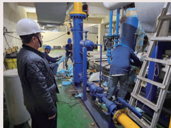
北館儲冰主機汰換 North Complex Ice Storage Host Replacement
