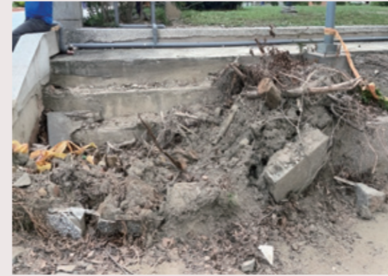
颱風致樹木傾倒損壞植栽矮擋牆 Typhoon caused trees to fall and damage planting low walls
